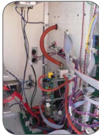
Figure 2: Internal Mass Flow Meter
